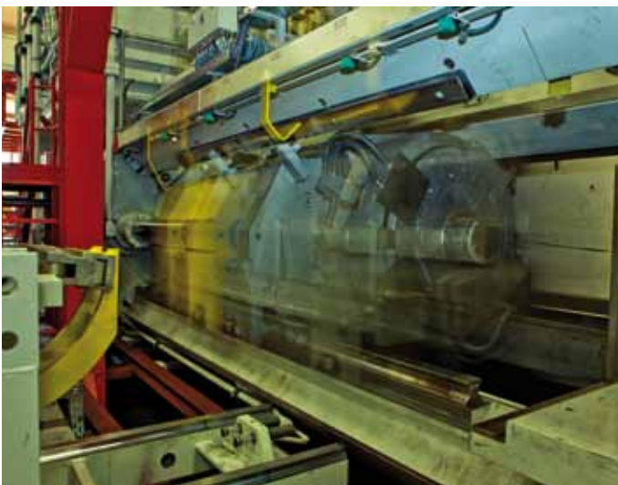
The new 35 MN extrusion press in Weissenburg, installed in 2011.
